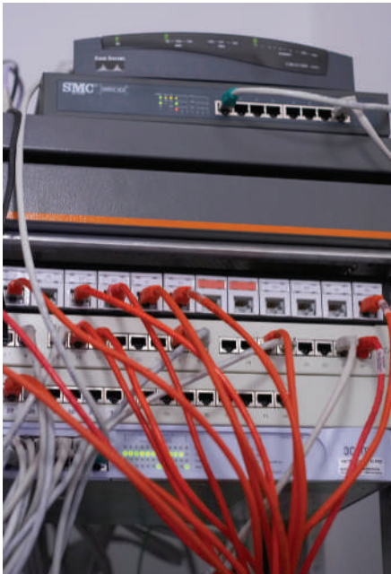
FIGURE 5-4 Networks use various devices that act like black boxes . Cables carry data in and out, but internal operations are hidden inside the case.
