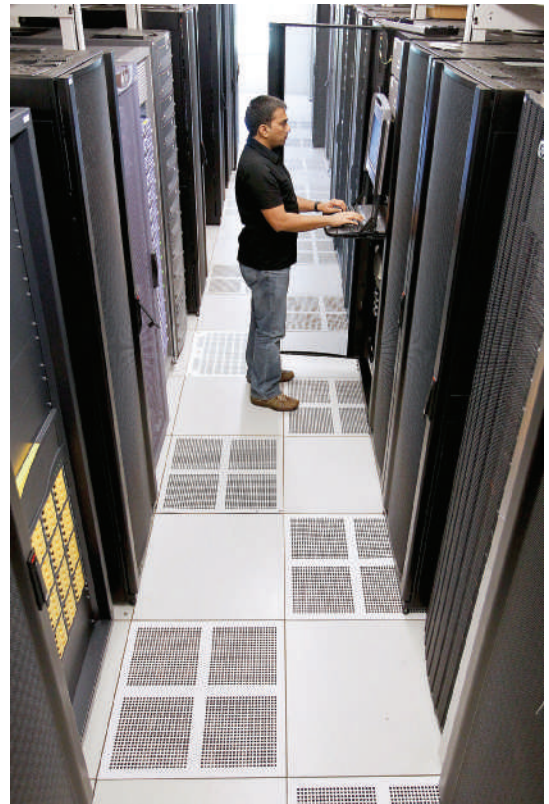
FIGURE 12-39 The rapid growth of data centers and server farms has increased energy consumption significantly and raised environmental concerns.
