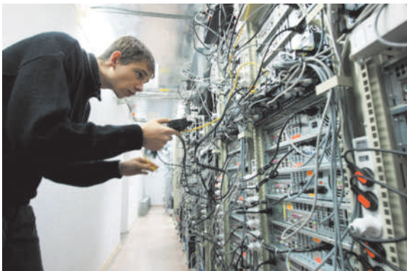
FIGURE 1-9 Multiple servers provide the power and speed that modern IT systems require.
